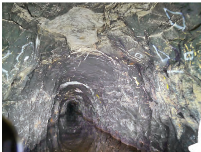
Rock-cut tunnel; visible on the ceiling are the long lines driven by the miners' hand drills. Photo Gerald Tompsett
